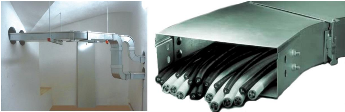
Fig 13: Non-perforated metal cable trays preventing re-emission from cables entering the protected premises from outside
