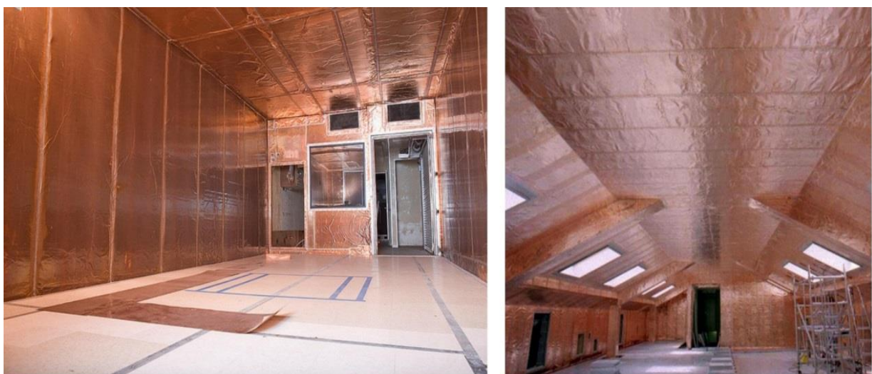
Fig 6: HEMP-protected premises lined with copper sheeting.
